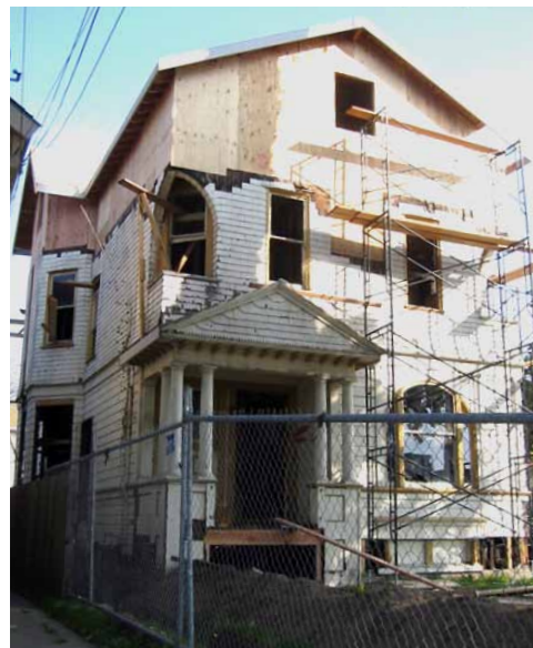
2007 photo showing initial reconstruction. Roof pitch is shallower than original, and second floor ceiling appears to have been lowered. (Photo: Patsy Baer.)
