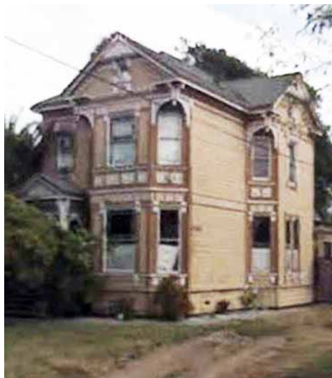
For many years the house suffered neglect and deferred maintenance. (Photo: Christina Yuen.)
