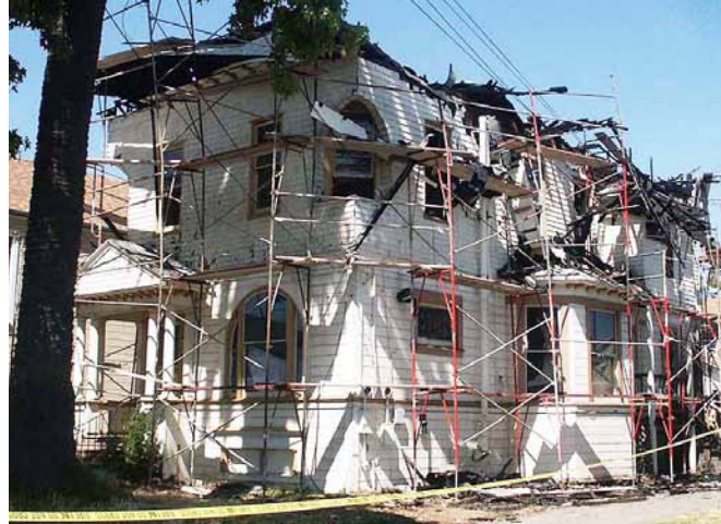
A 2006 photo showing the aftermath of fire, with roof and attic completely destroyed.
