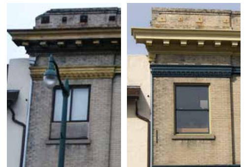
Left: During the 1970s two wooden windows were replaced by shorter aluminum ones, finished off with faux brick contact paper.
