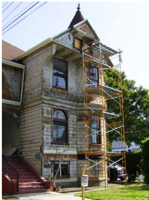
José Puicon did all of the interior painting, and single handedly prepared and painted the exterior.
