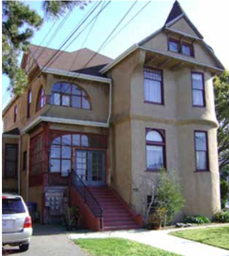
For 50 years the mansion was encased until John Jameson removed it with a hand-held circular saw so not to damage the original siding..
