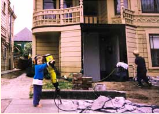
The stairs with metal railing and part of the porch had to be removed. Robert's son displays his talents with the jack hammer. Images: Farrar family collection. (circa 1998)
