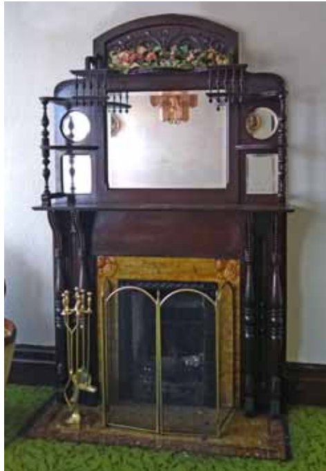
Original fireplace mantle before restoration – note thick dark finish with streaks and cracking.
