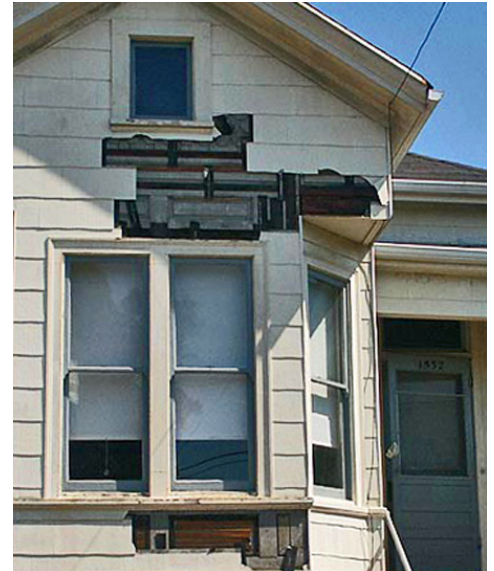
Modern siding being removed from a home to show original millwork hidden beneath.
