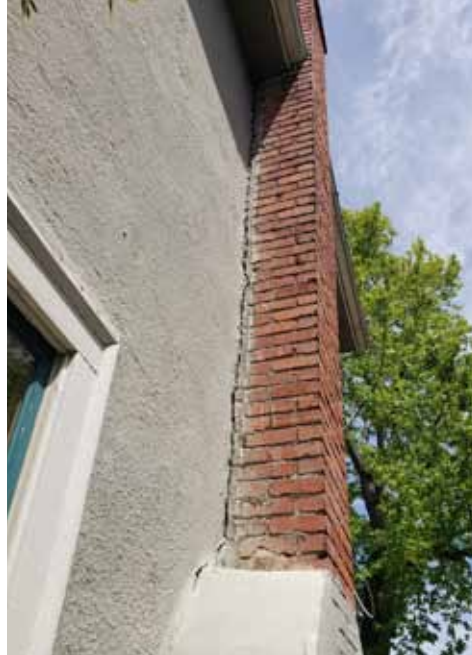
Chimney pulling away from house. Image: Jason Wady.
