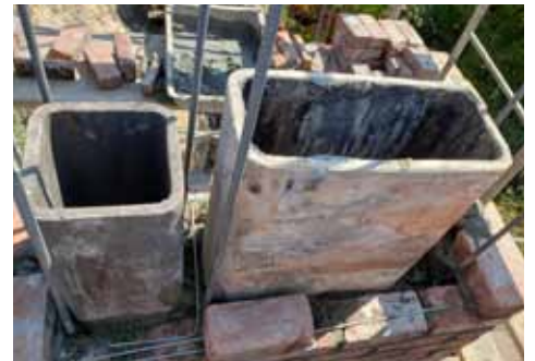
Installation of the existing cleaned bricks with wire and rebar reinforcement. Image: Jason Wady.
