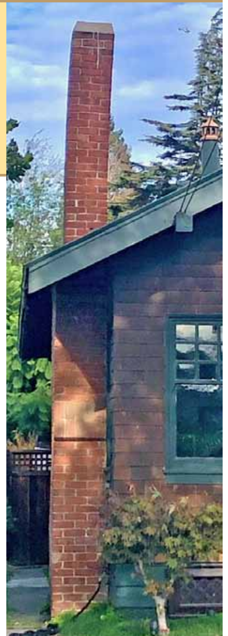
Leaning chimney in East End Alameda. Image: Karen Lithgow.
