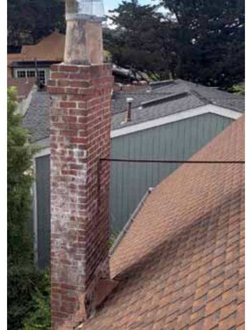
A rebar holding the chimney. Image: Jason Wady.
