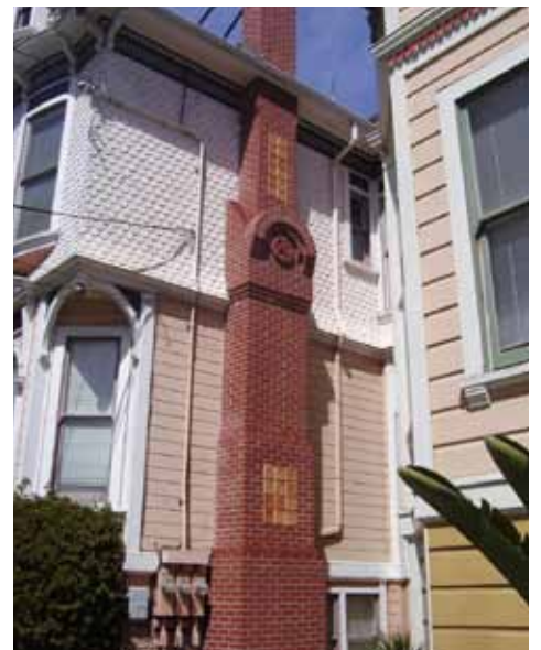
This chimney has a unique design with ceramic tile inlays. Image: Hans Thiering Masonry.
