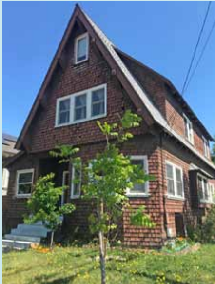
Notice the long dark brown boards are covering the front of the brackets. There are also multiple shingles missing all over the front facade and discoloration under the top window.
