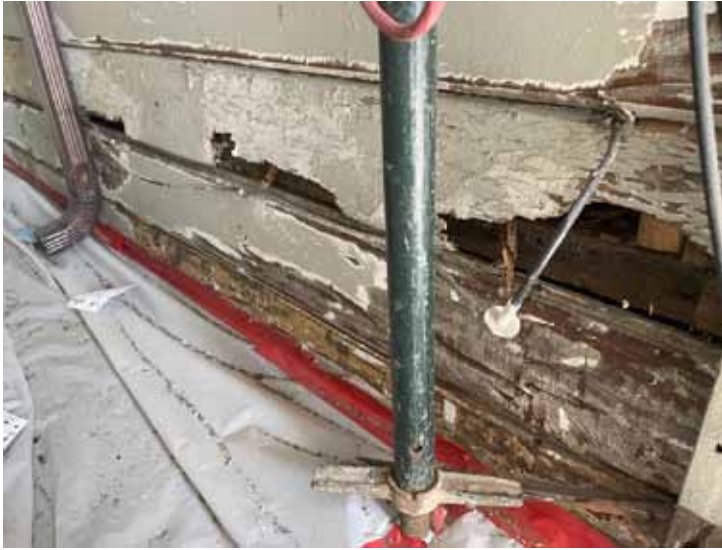
Here is an example of dry rot. These boards must be removed and replaced. Image: Myron Olson.
