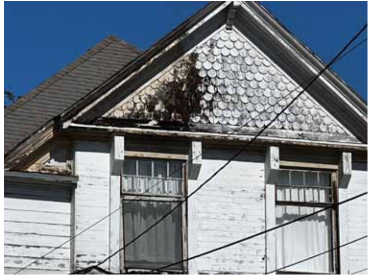
Here's an example of dry rot causing structural damage underneath. Image: Devon Westerholm.
