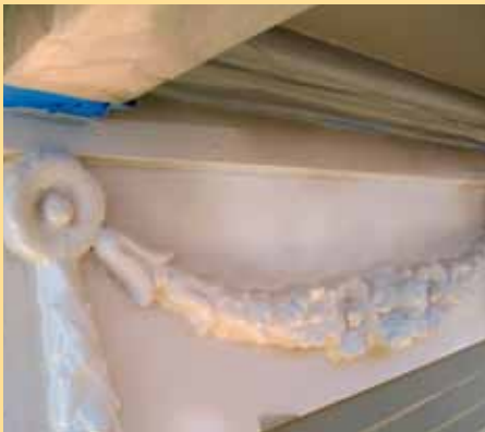
Some of the original plaster pieces were missing and had to be recreated.
