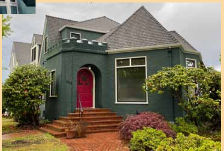
The roof was raised, dormer windows incorporated and half-timbering on the exterior walls in keeping with the original architectural design were added. However, by not expanding the entry and front room, the house retains its original look and creates the illusion that it remains unchanged.
