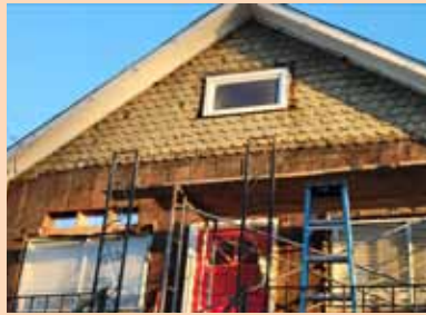
Beneath the layers remnants of the original scalloped shingles were uncovered and re-incorporated into the final design.
